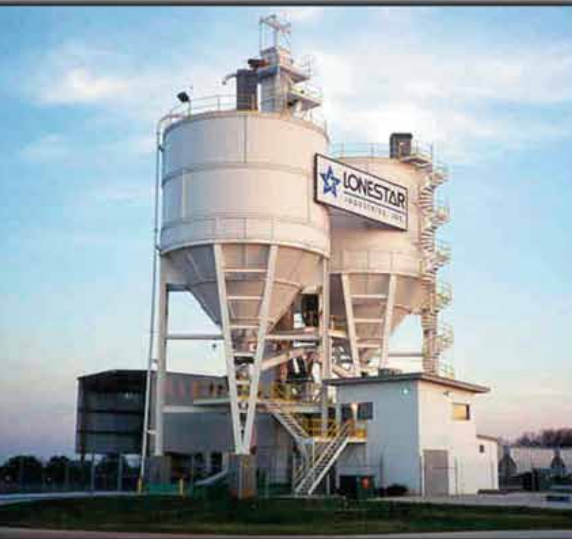
35' diameter terminal silos
