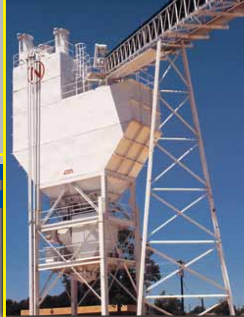
Weigh hopper under "SB" style aggregate bin
