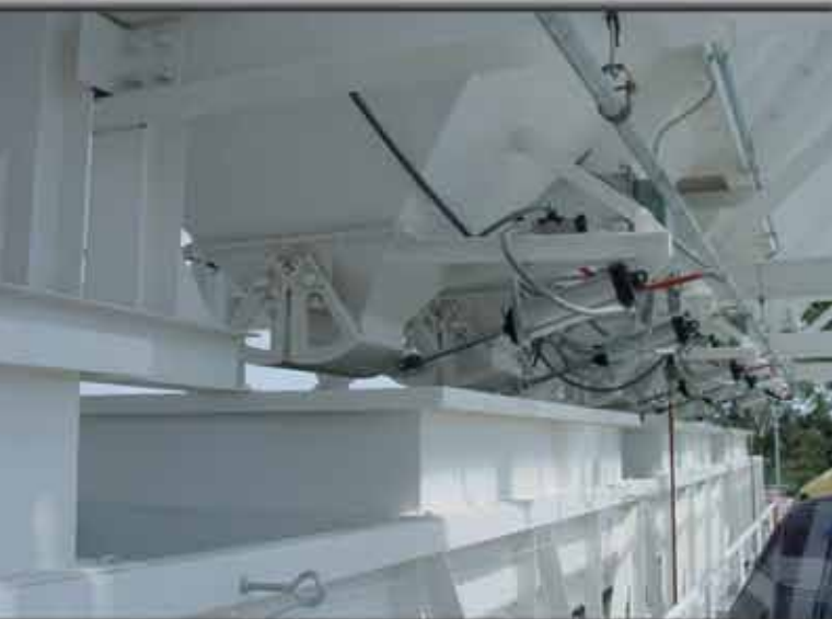
Aggregate bin gate bottom and weigh belt conveyor
